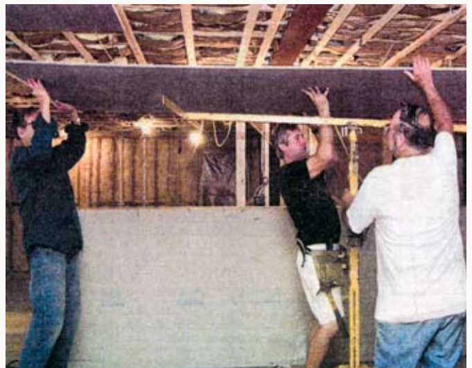
Soderholm Carpentry Inc, workers put up “blue board at a construction site last week.
